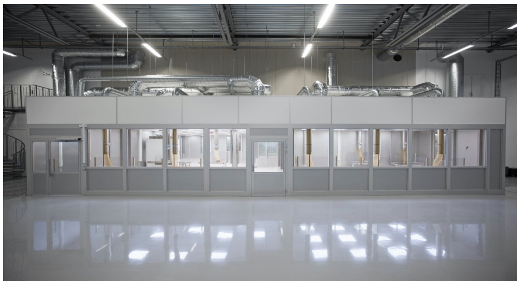
Cleanroom at APL
